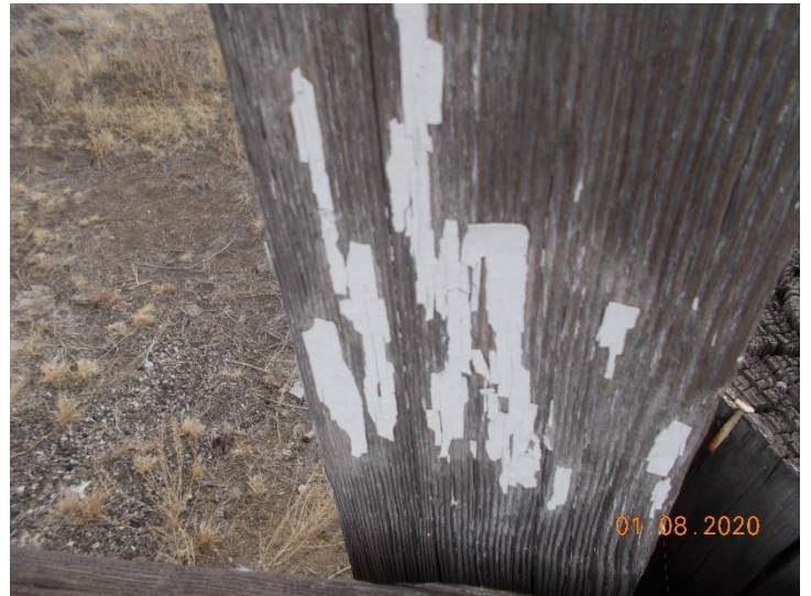
Paint sample N-21-F-LP01. The white paint is considered as lead containing paint.
